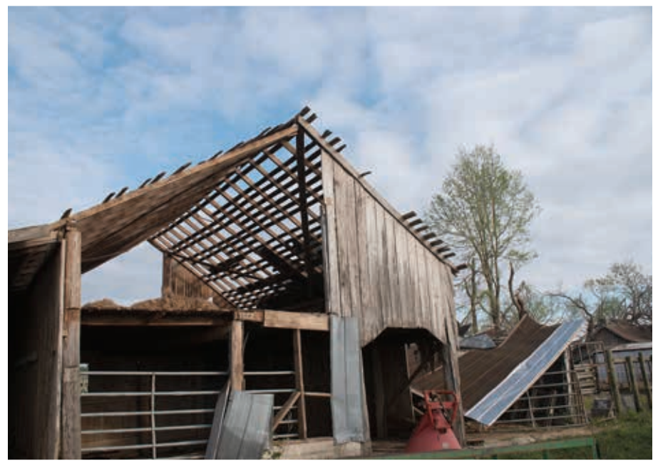
Above: Hurricane Michael damaged buildings, corrals and fences on John Hill’s operation.
