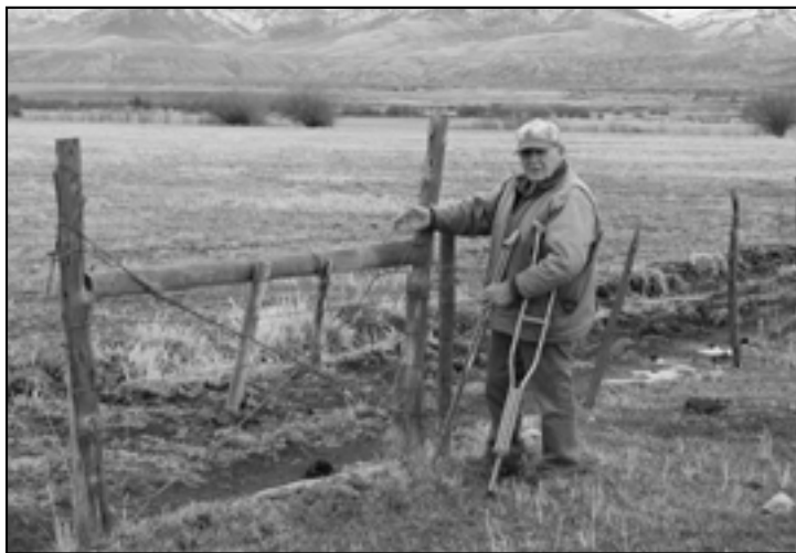
Photo 1: Jack Walther says most braces are incorrectly constructed with the crosswire attached to the opposite post at a height above the horizontal cross member.
