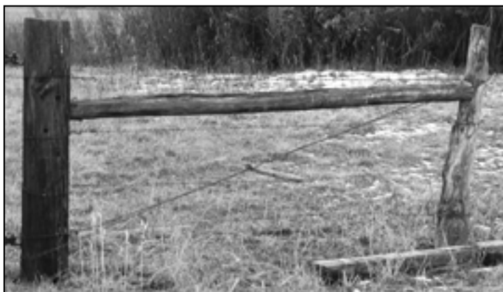
Photo 2: A properly constructed H-brace has the diagonal crosswire at the same height as the horizontal cross brace.
