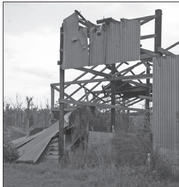
Pomes' horse barn is in ruins after Hurricane Katrina filled it with 8 feet of water.
