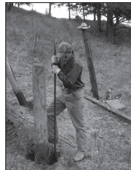
IX Ranch Co. interns take part in all ranching activities, including building fence. [PHOTO COURTESY IX RANCH CO.]
